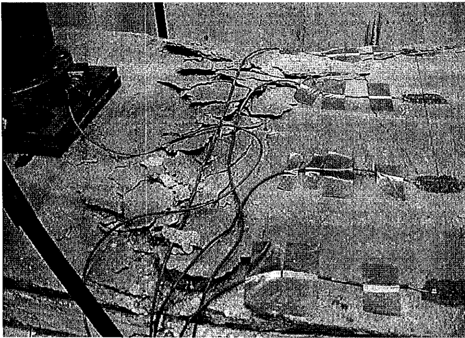
Figure 4.5. Line of ruptured concrete across the deck of Cedar 1.
