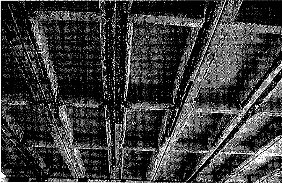
Figure 3.20. Bridge 3 corrosion damage.
