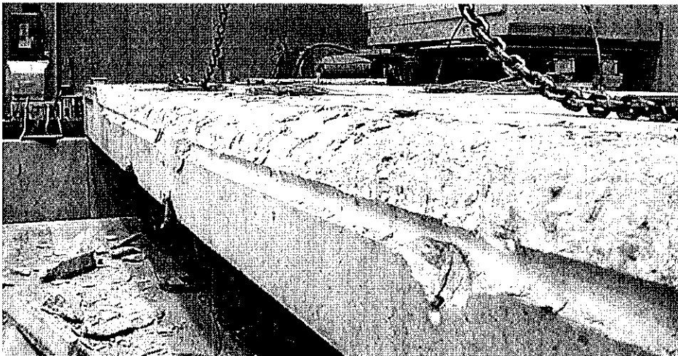
Figure 5.13. Failed concrete above shear connector in P3 (looking east).
